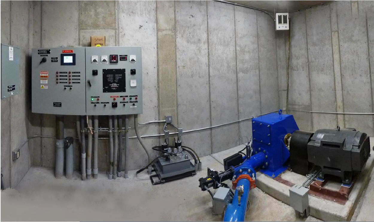
FIGURE 2 – PHOTO OF PELTON GENERATOR AND CONTROLS
