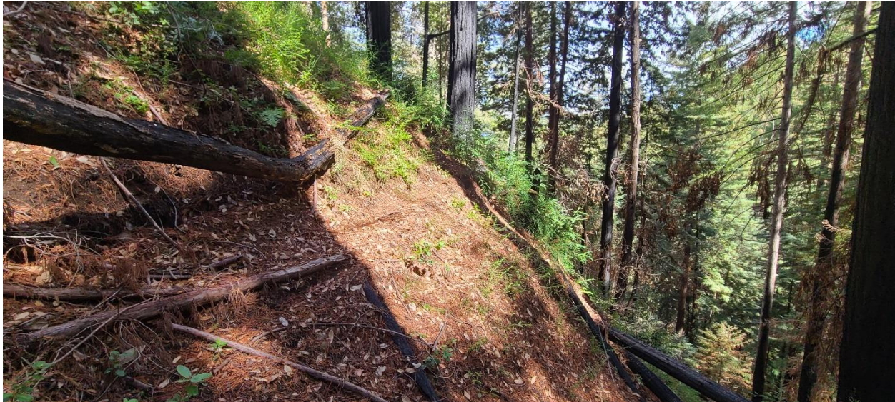
Photograph 10: Example of Extremely Steep Slope and Outboard Slope Failure along Existing Waterline Bench
