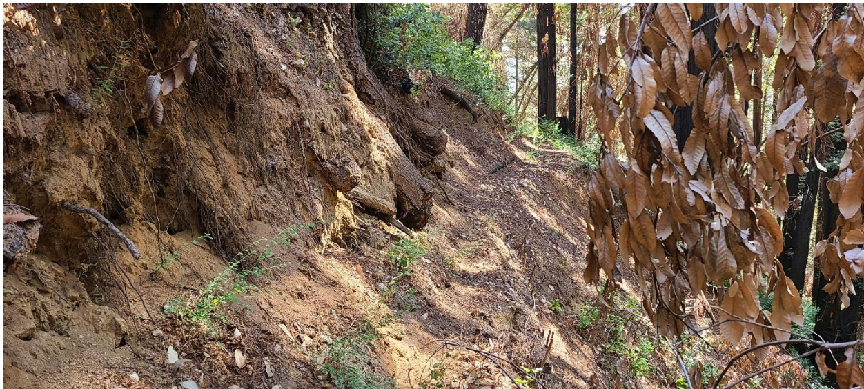
Photograph 7: Example of Extremely Steep Slopes, Unstable Conditions and Large Root Wad Along Existing Waterline Bench
