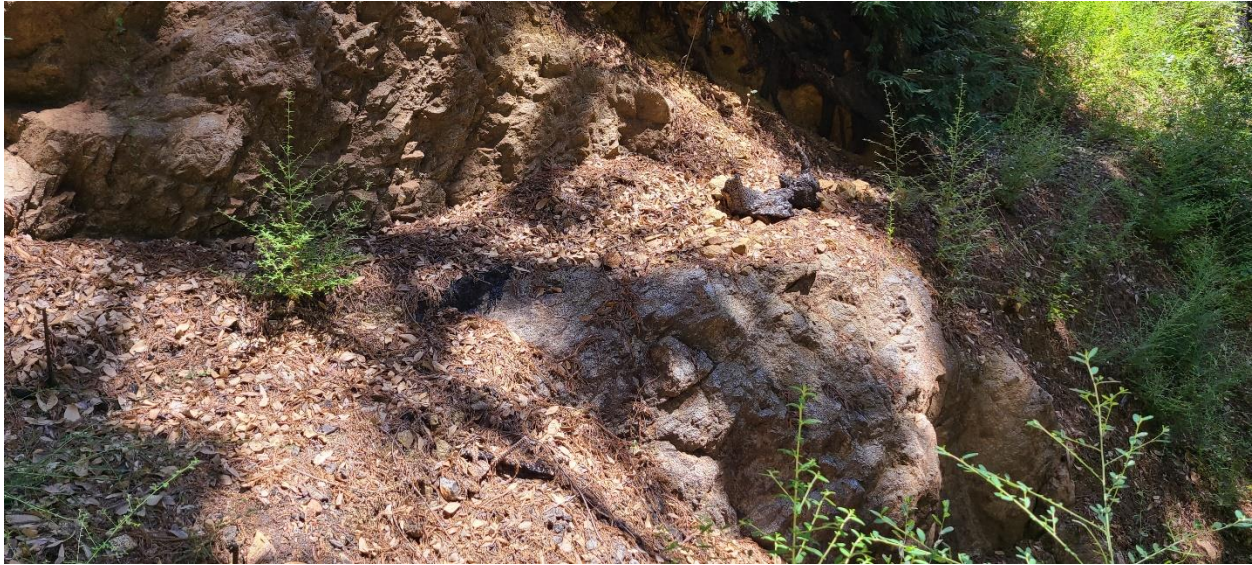
Photograph 1: Example of Extremely Steep Slopes Along Existing Waterline Bench at North side of Clear Creek #1 crossing
