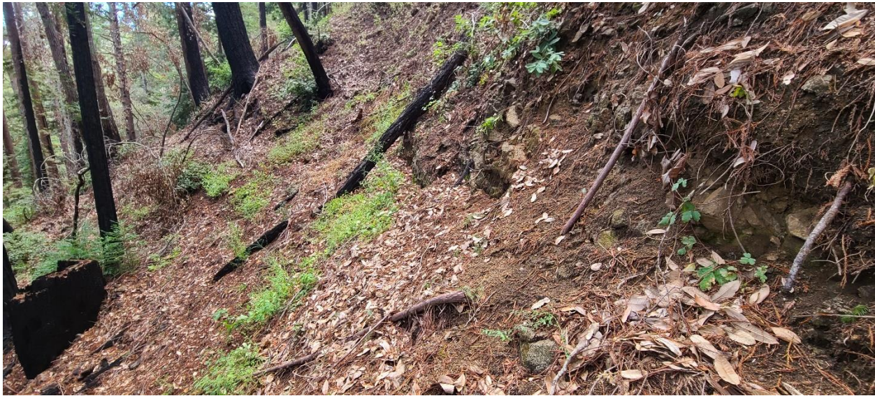
Photograph 8: Example of Steep Failing Slopes along Existing Waterline Bench
