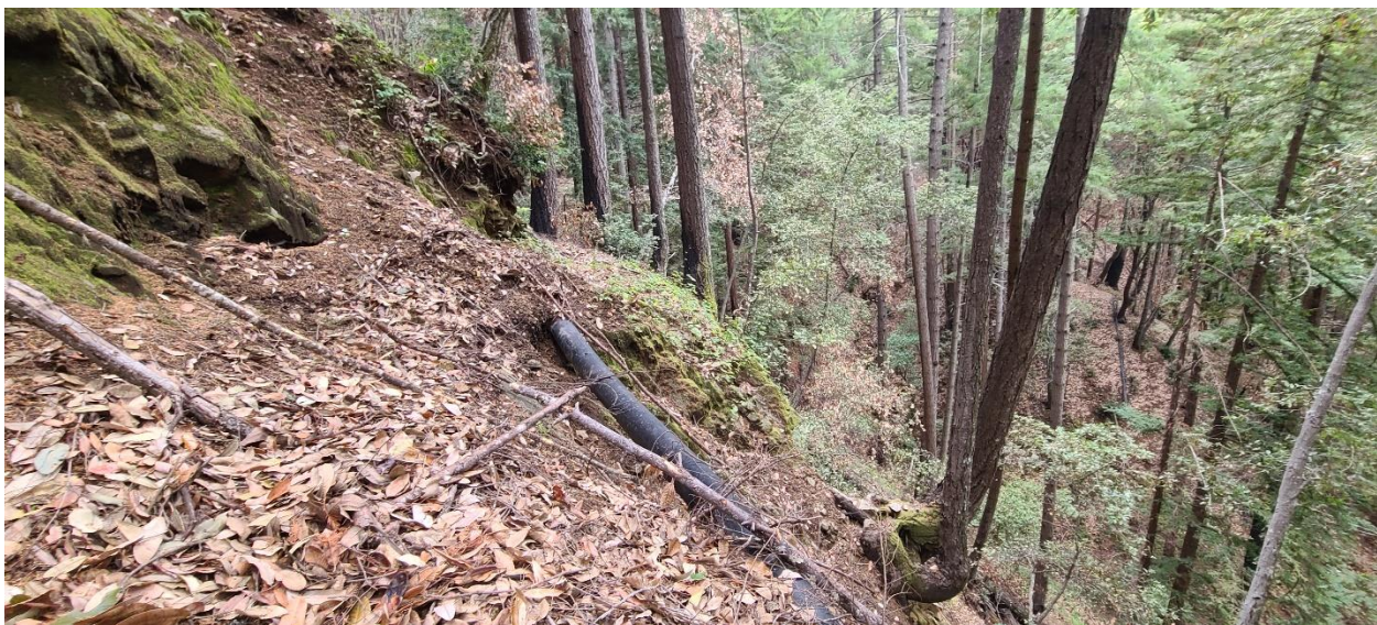
Photograph 2: Example of Extremely Steep Slopes Along Existing Waterline Bench with Black HDPE Pipeline Visible
