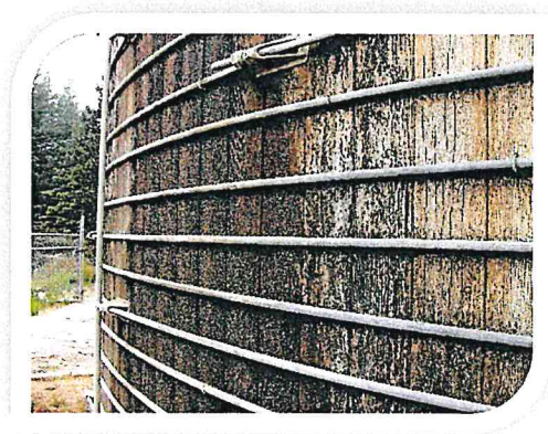
Lewis Tank, Wood Stave Condition
