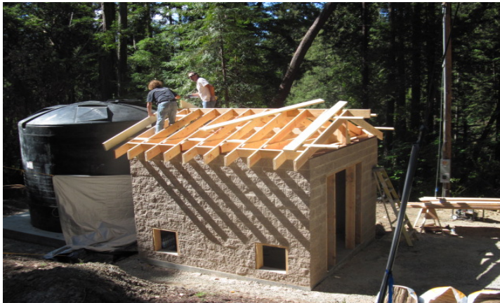
Pump house in Zayante
