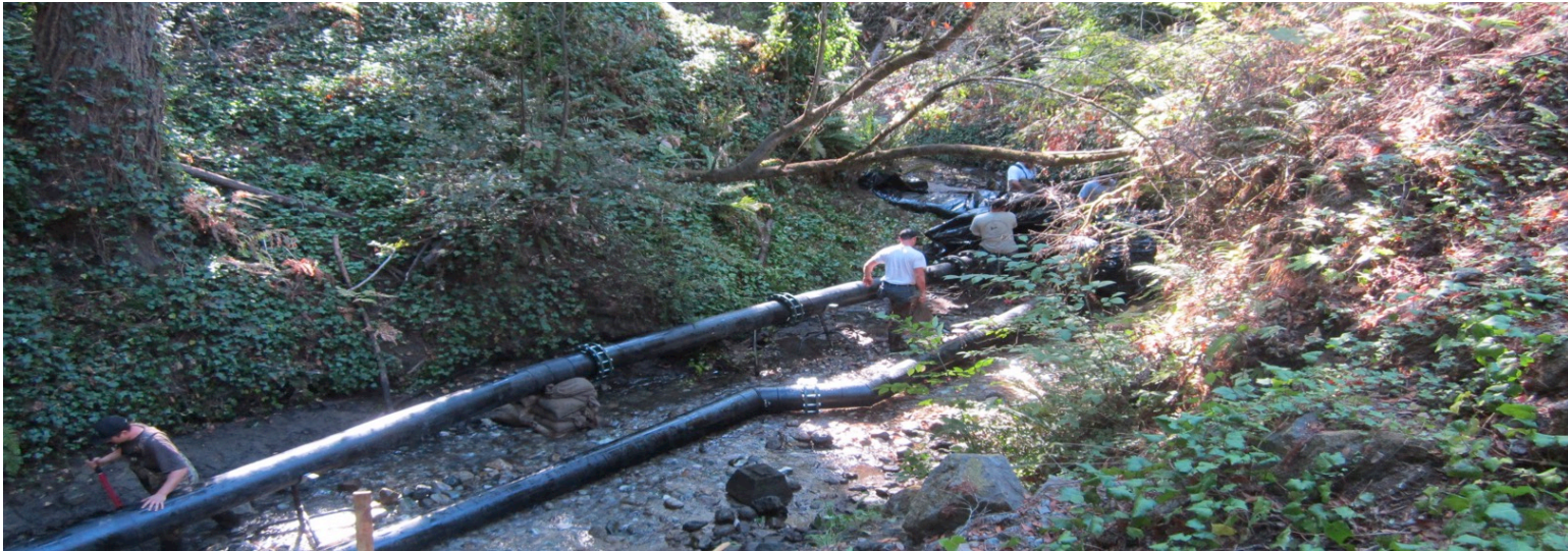
Fall Creek Temporary Bypass Pipeline
