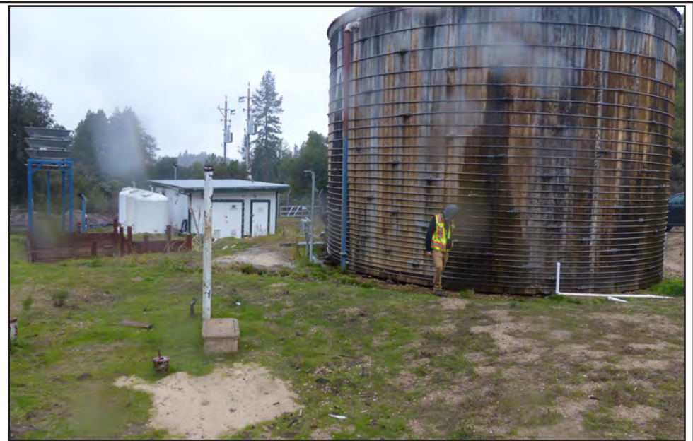
Photo 2. View of Lewis tank site looking south, showing the existing leaky redwood tank and abandoned water treatment infrastructure.
