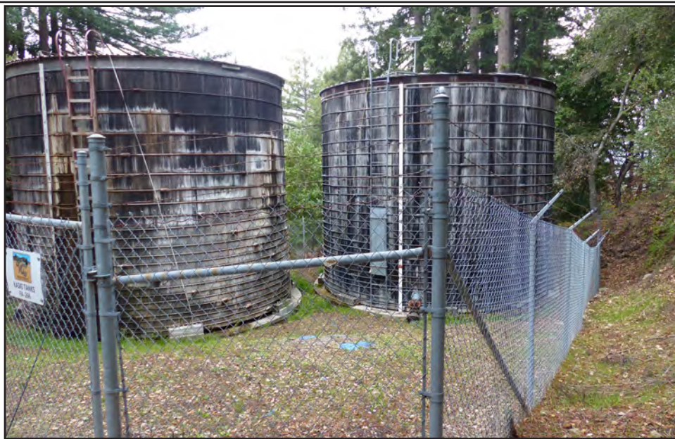
Photo 1. View of Kaski tank site looking southwest, showing the existing leaky redwood tanks.
