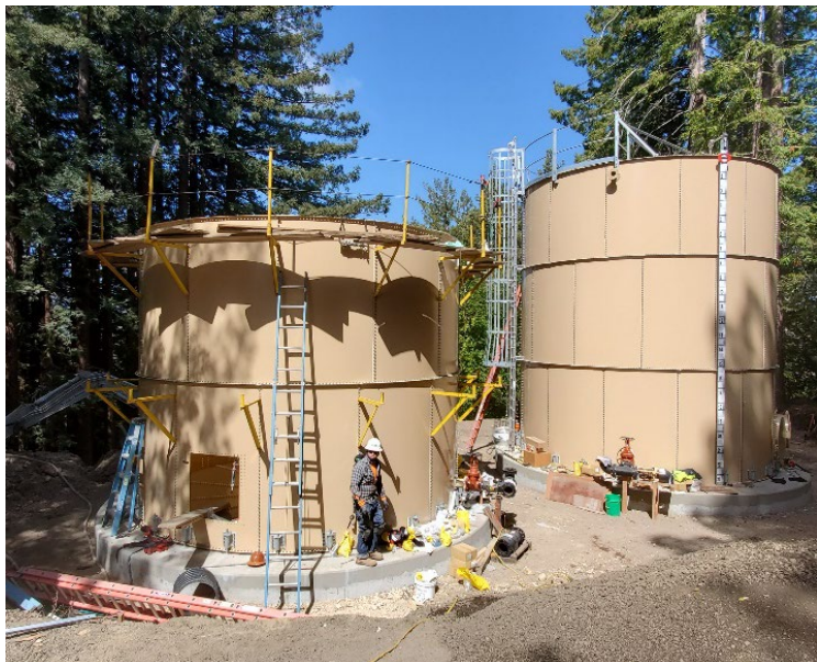
Kaski Site – Twin 42,000 gallon tanks, 20' Ø, 23' H
