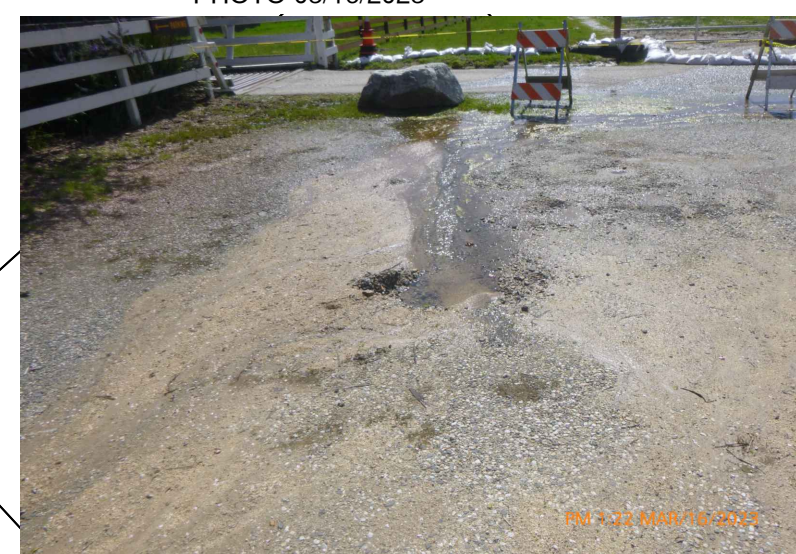
QUAIL HOLLOW RANCH PARKING LOT CLOSED HIGH WATER TABLE PHOTO 03/16/2023
