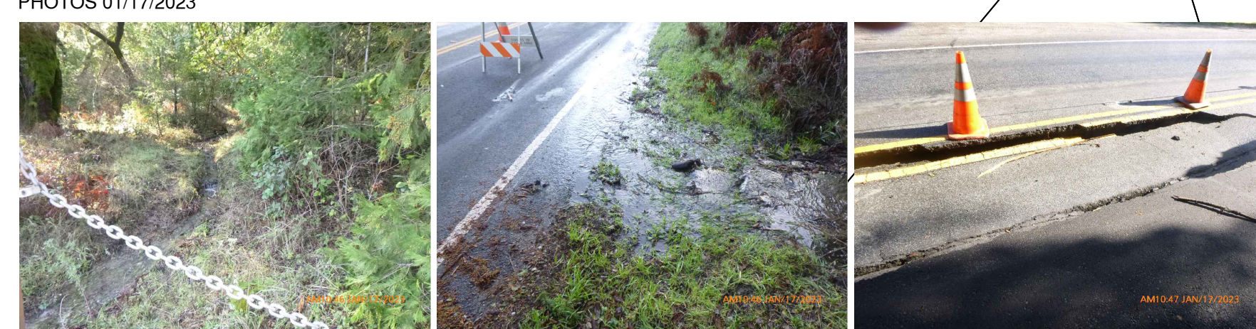
JANUARY STORM DAMAGE REPAIRED BY SANTA CRUZ COUNTY PUBLIC WORKS DEPARTMENT & GRANITEROCK PHOTOS 01/17/2023
