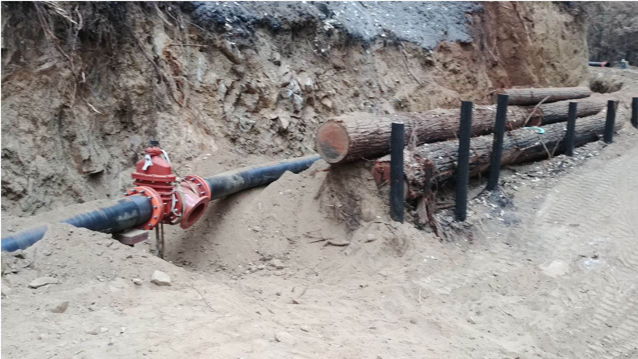
Figure 3: Blowoff at access road on Foreman pipeline
