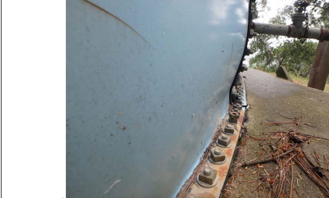
Structural Sidewall buckling possible due to an earthquake.
