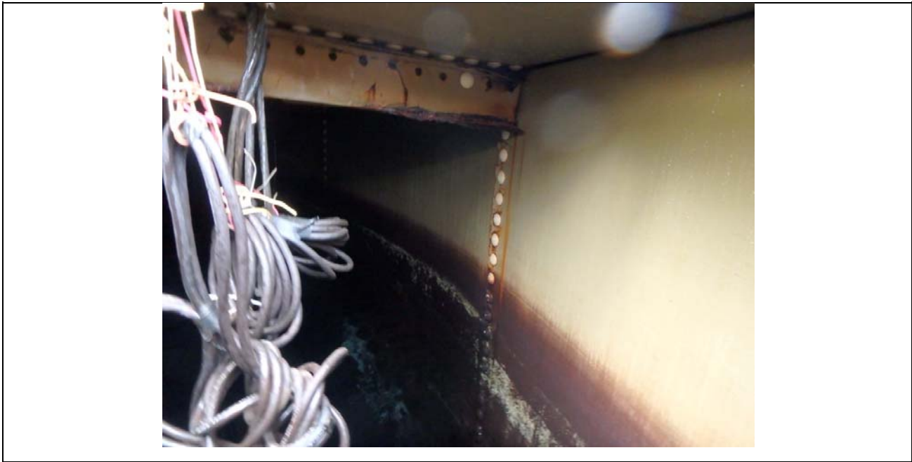
Structural - Roof Structure Heavy rusting and corrosion.
