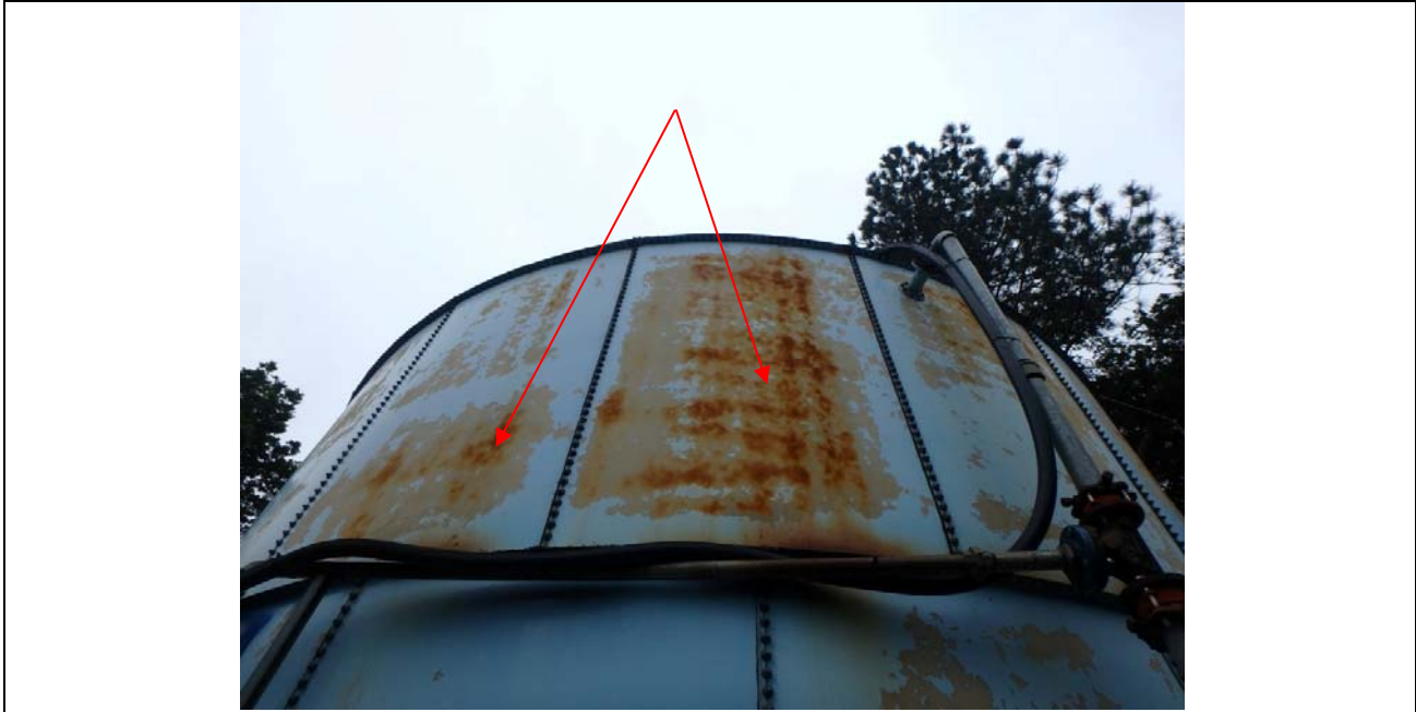
Exterior Coatings Example of rust sites on shell.
