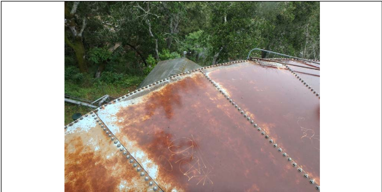
Exterior Coatings Sever corrosion on roof.
