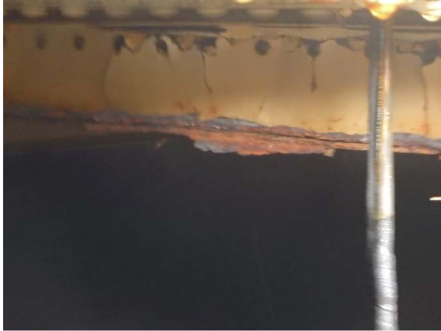
Structural - Roof Structure Heavy rusting and corrosion.
