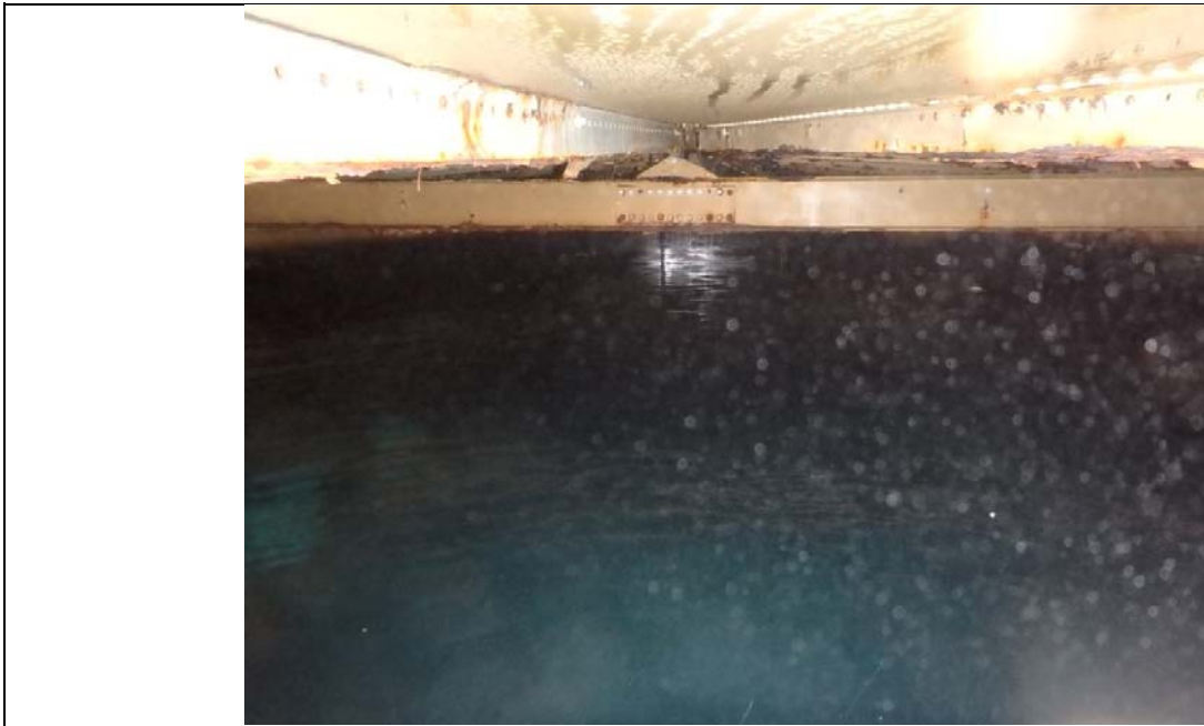
Structural - Roof Structure Heavy rusting and corrosion.
