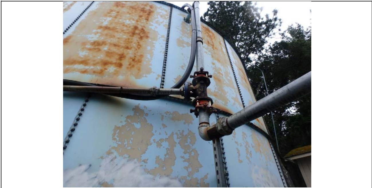
Exterior Coatings Corrosion on shell.
