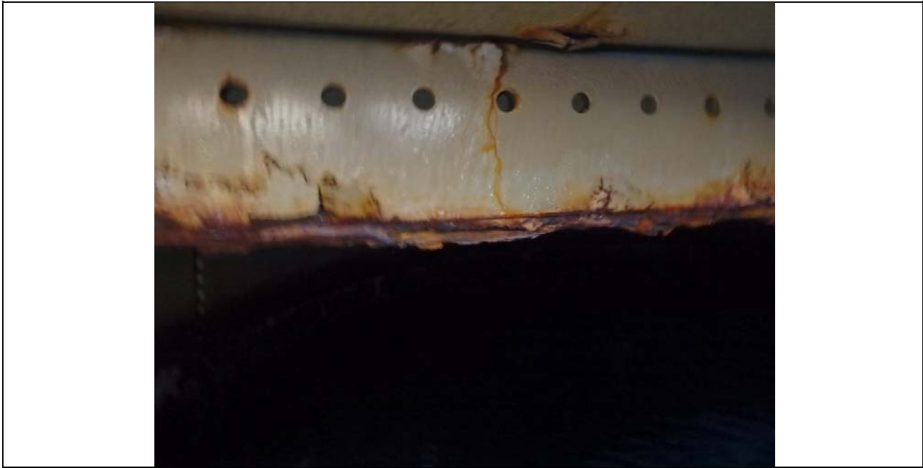
Structural - Roof Structure Heavy rusting and corrosion.
