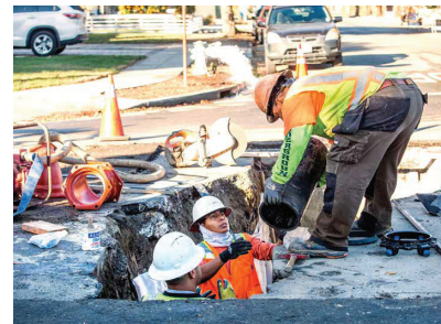
Maintaining the City's infrastructure includes repairing or replacing water mains due to age or condition.
