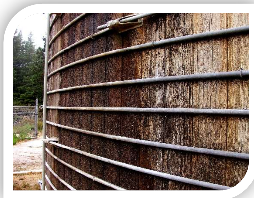
Lewis Tank, Wood Stave Condition
