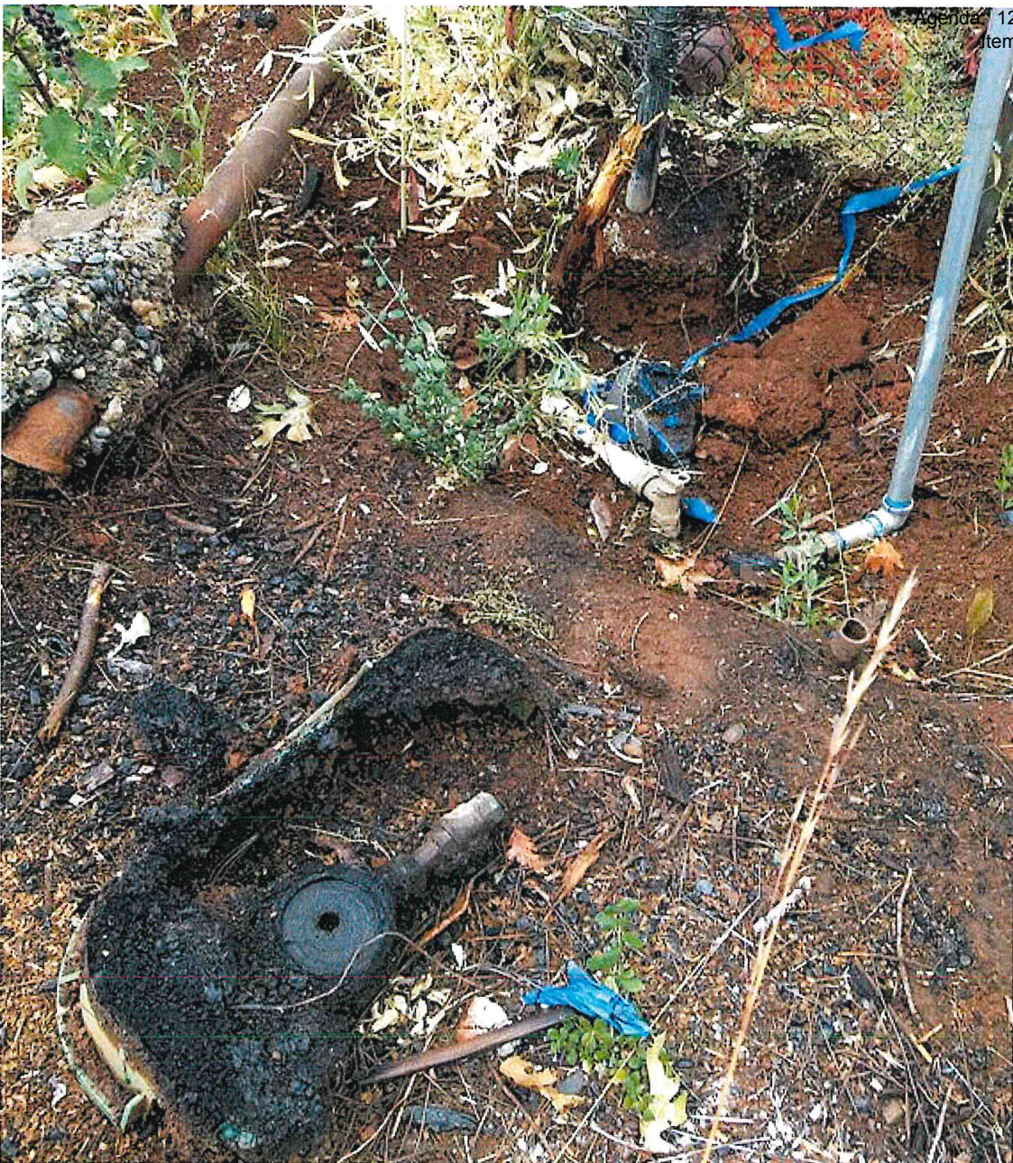
Damaged water meters like this one photographed in Paradise, California, after a wildfire swept through 2019, can release volatile organic compounds, potentially contaminating drinking water. Photo courtesy of Gina Solomon
