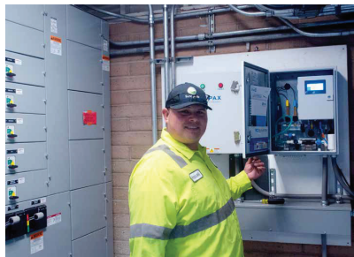
Senior Water Distribution Worker Manuel Hernandez checks water pressure and chlorine levels at the City's pump stations.
