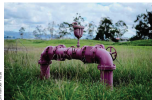
Recycled water represents 3% of the City's total water supply. We have been producing recycled water since 1993. We currently deliver it to 120 customers for non-potable uses such as cooling towers and irrigation.
