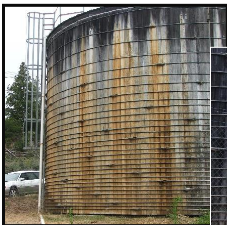
Lewis Tank One
