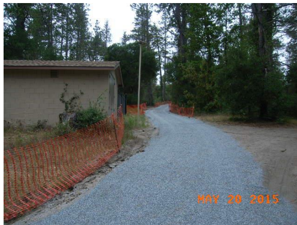
Figure 6B. View of existing paved access road between Graham Hill Road and Probation Tank, near existing SLVWD pump station, looking northerly.
