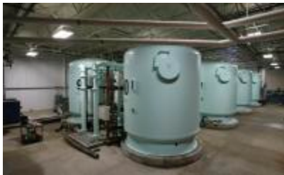
This Wednesday, July 15, 2015 photo shows tanks in the Nitrate Removal Facility at the Des Moines Water Works plant in Des Moines, Iowa. The biggest
