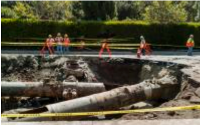
FILE - In this Thursday, July 31, 2014 file photo, Los Angeles Department of Water and Power crews work to repair a juncture of a water main which ruptured
