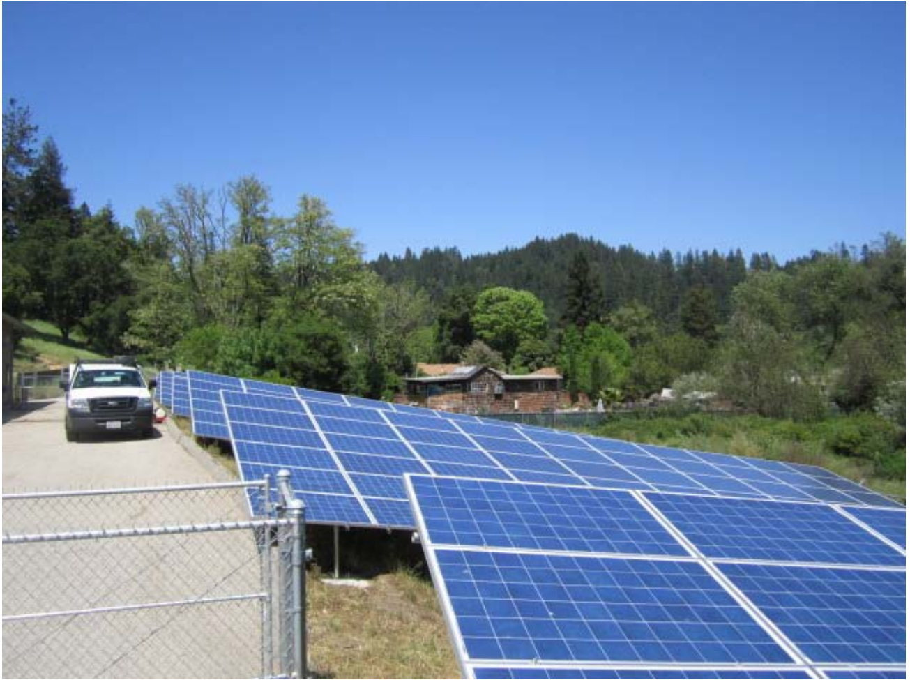
San Lorenzo Valley Water District's new solar installation at the Kirby Street water treatment plant in Felton, to be showcased at an open house Friday, August 26 at 3:00 p.m.
