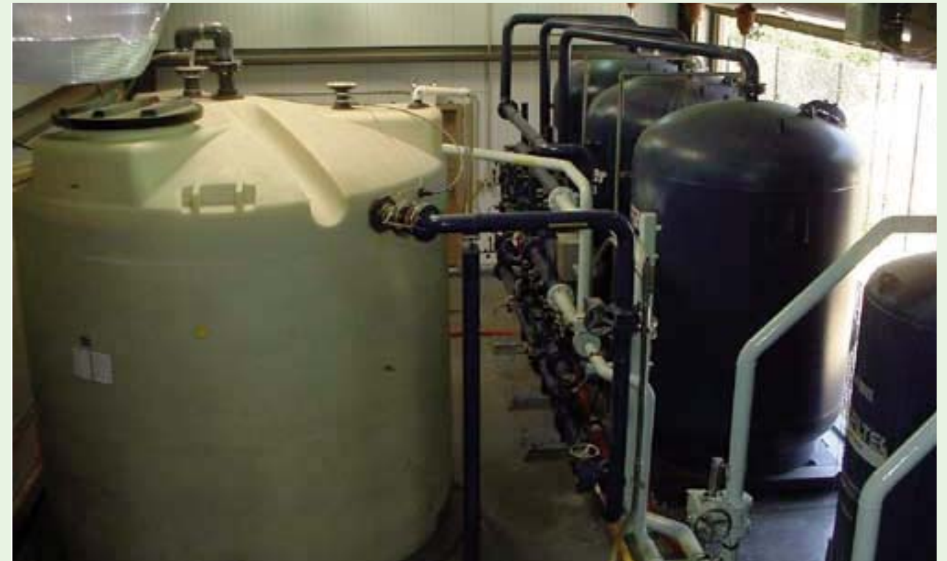
Manana Woods Water Treatment Facility
