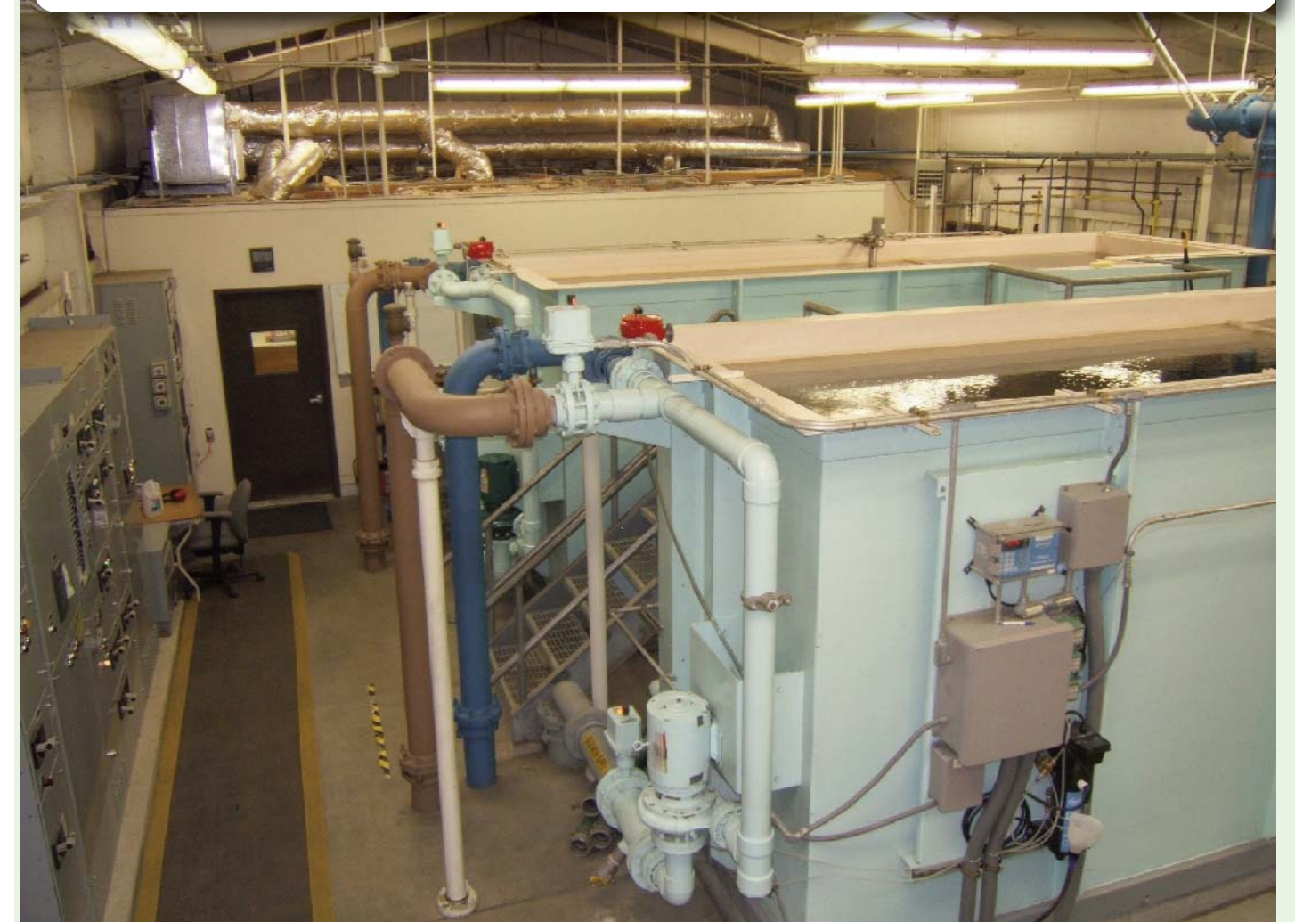
Kirby Street Water Treatment Plant. Water filtering units #1 & #2, combined these two filter units have the ability to treat and filter 720 gallons per minute or 1.3 million gallons per day for the 1,300 residents of the Felton water distribution system
